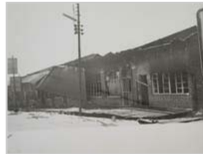
Hostel, partially collapsed roof.
